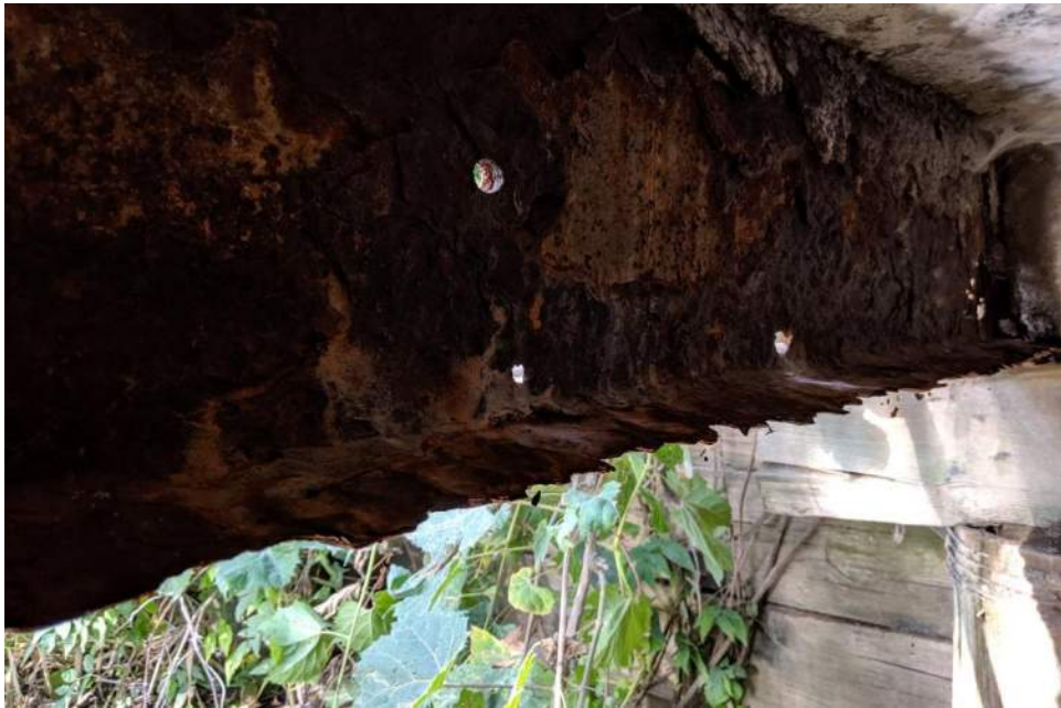
South Fascia Beam Deterioration
