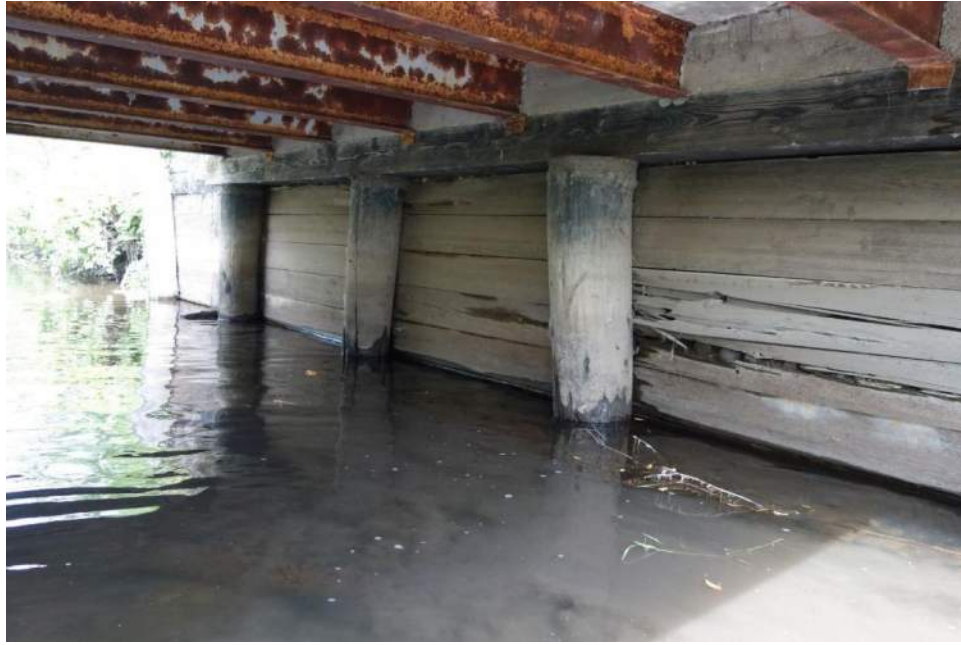
Typical East Abutment Deterioration
