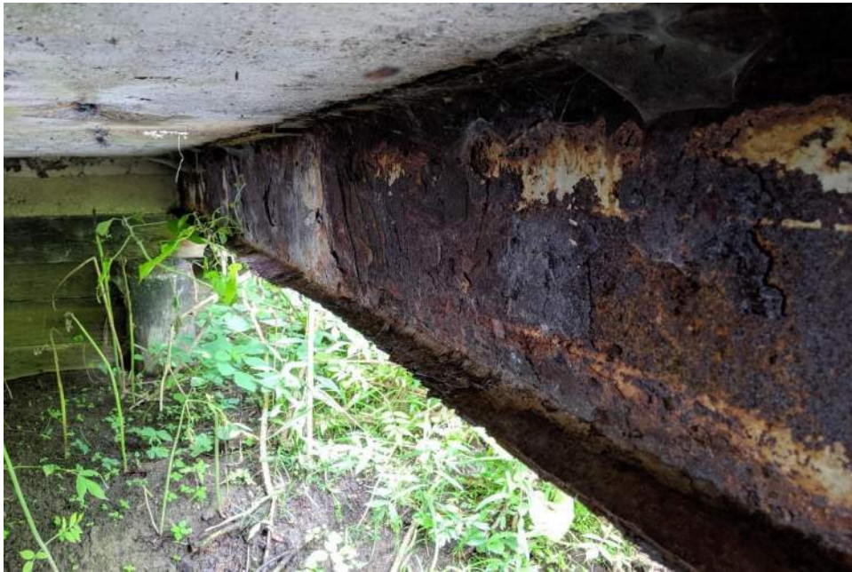
North Fascia Beam Deterioration
