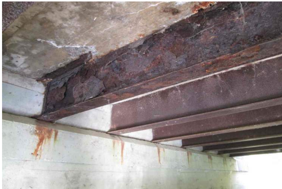
Beam 3 South with Section Loss
