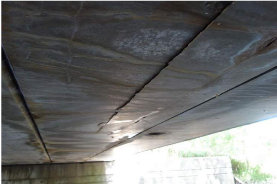
Beam 10W Cracking and Delamination
