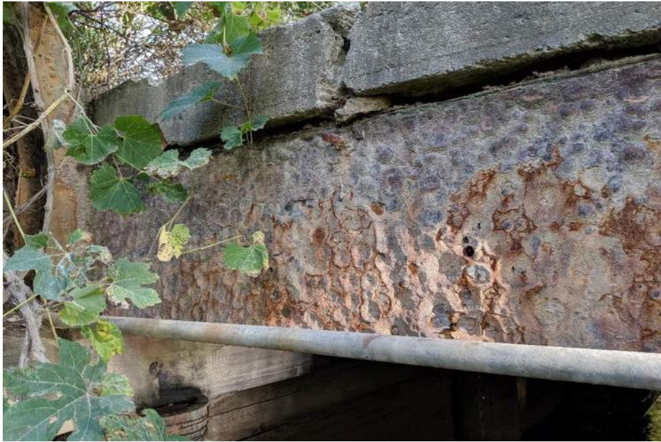
South Fascia Beam Deterioration
