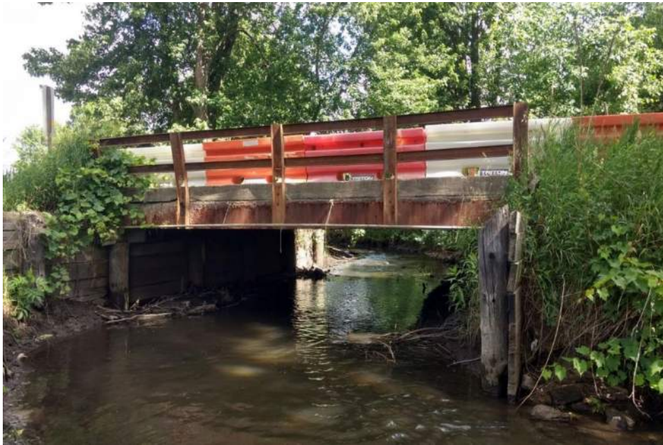
South Elevation and Poor Channel Alignment
