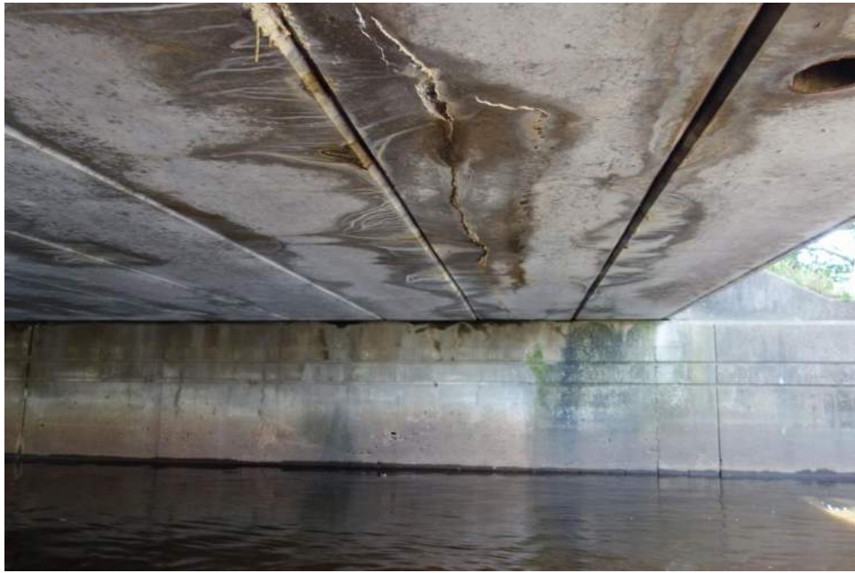
Beam 2W Cracking and Delamination
