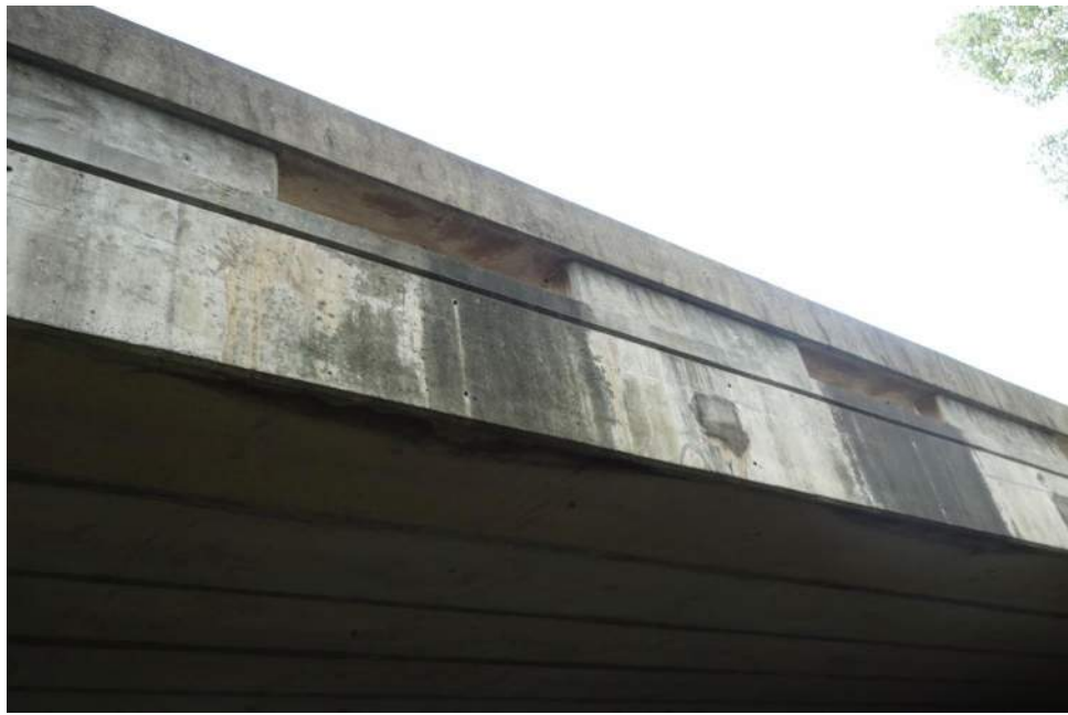
Fascia Showing Water Staining from Over Fascia Drainage
