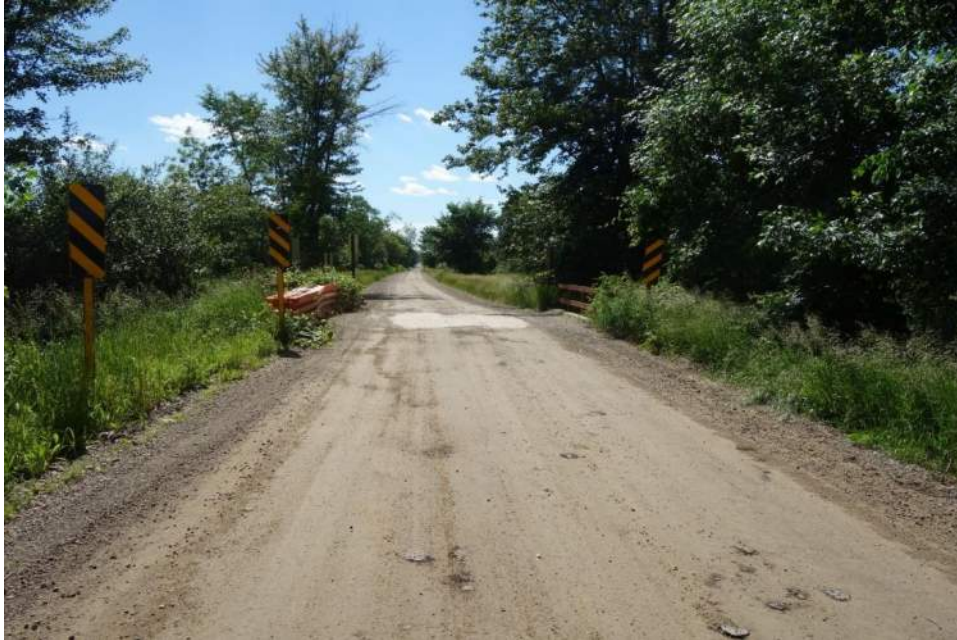
Approach Looking West (note temporary barrier to keep load off fascia beam)
