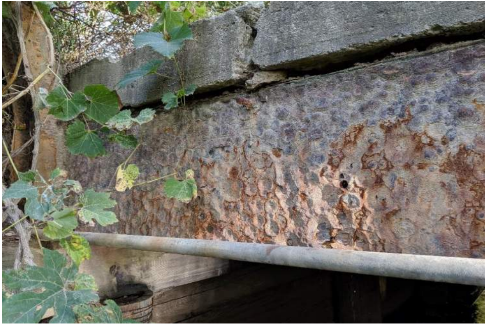
South Fascia Beam Deterioration
